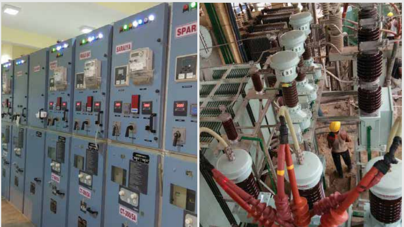
Project : Integrated Power Development Scheme (IPDS) - Varanasi
